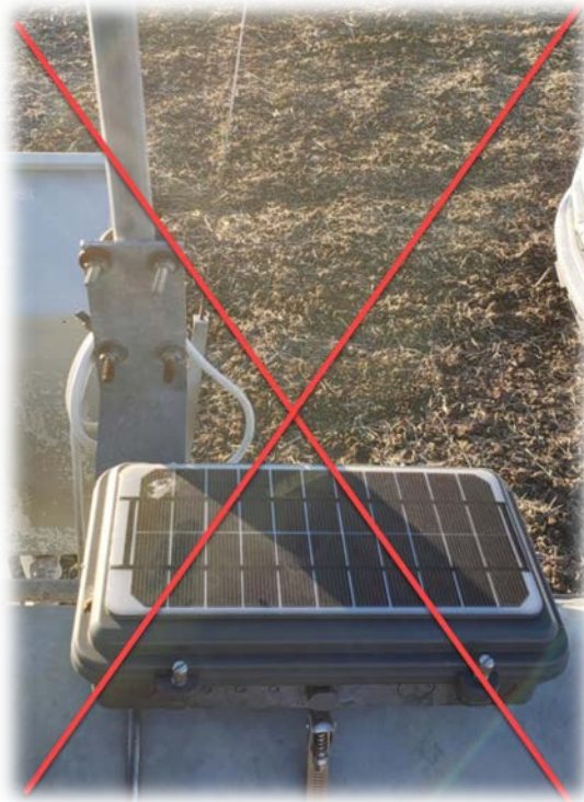
Overhang is obstructing sunlight
