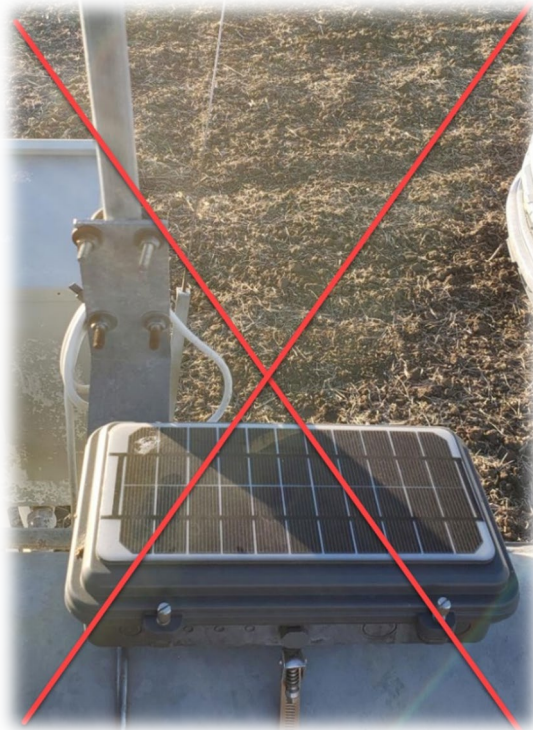
Overhang is obstructing sunlight
